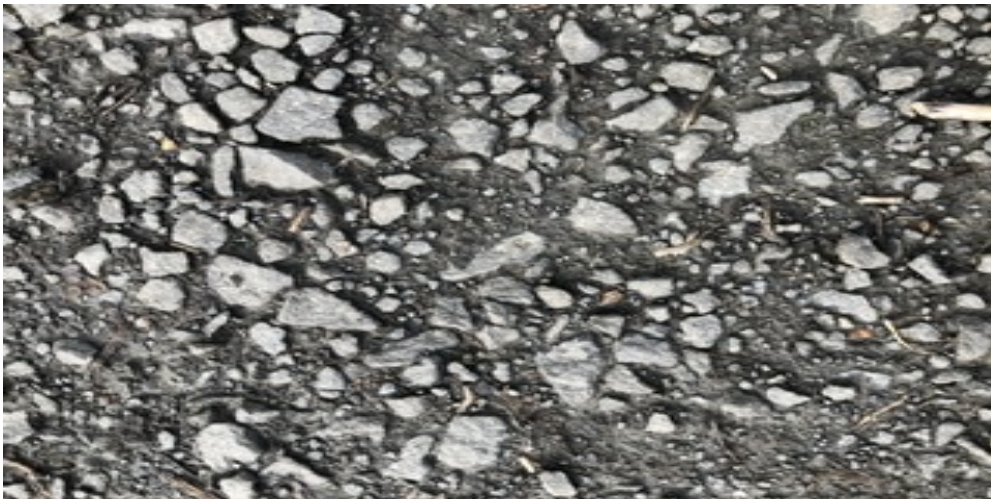
Location: almost everywhere where the path is dry. Shows how the path has been reduced to bare metal from sheer wear and tear; it has not been renewed since it was built as part of the Millennium Project in 2001.
