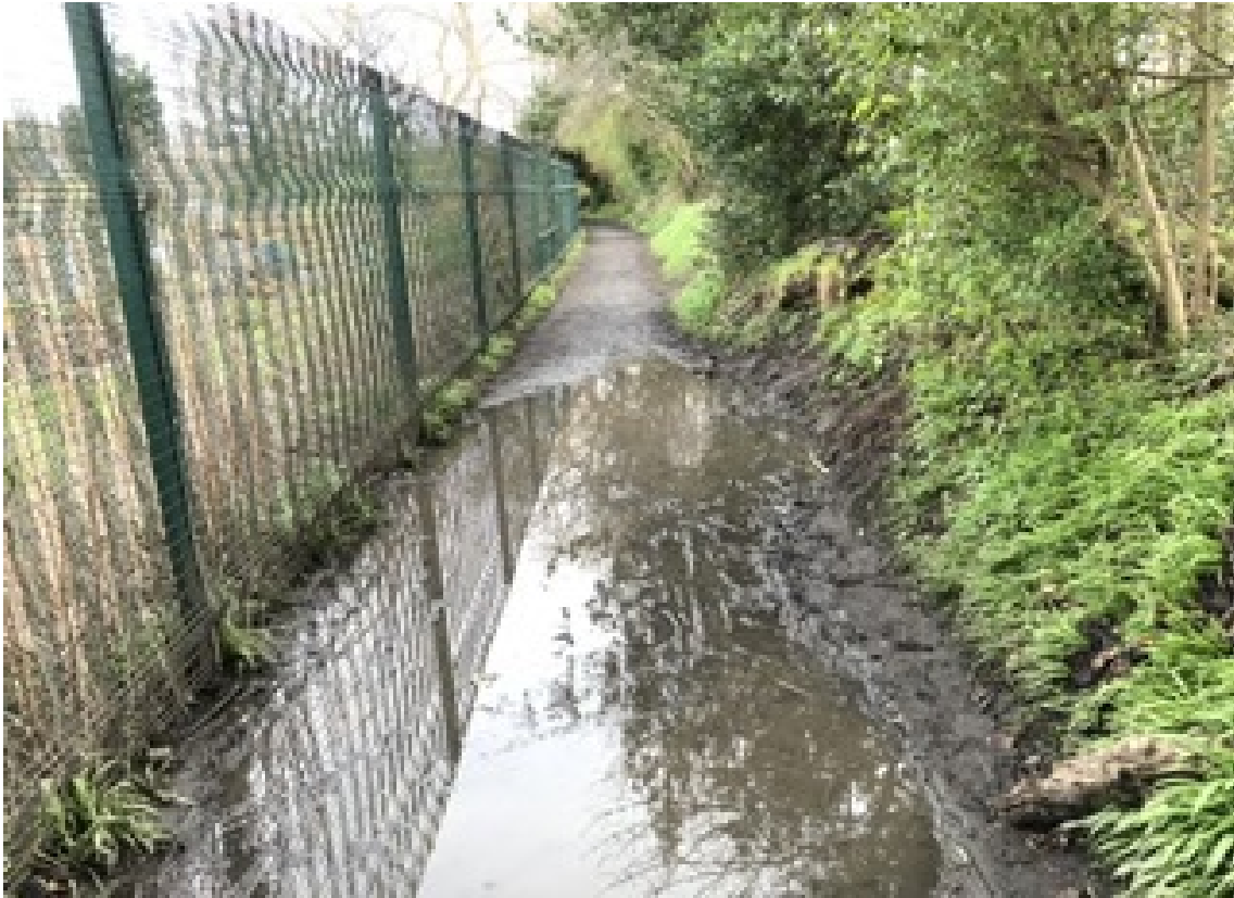
Location: Saughton allotments. Notice how, here and in the other photos, the path has “spread” along the edges as users try to avoid the water. At this particular spot the puddle is so long that users have gone over the bank and diverted to an informal 'fisherman's' path closer to the river.
