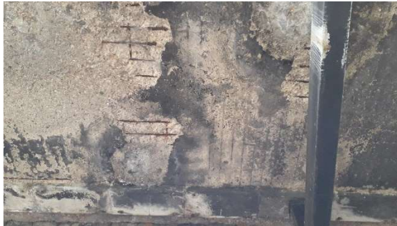
Figure 1 Degraded concrete and exposed steelwork
