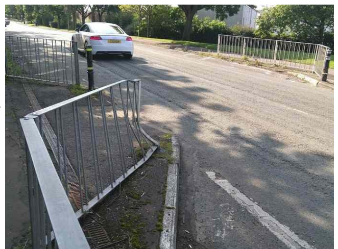
The existing un-signalled crossing is 6 meters across, shows significant impact damage and is inadequate as a safe route to a primary school.
