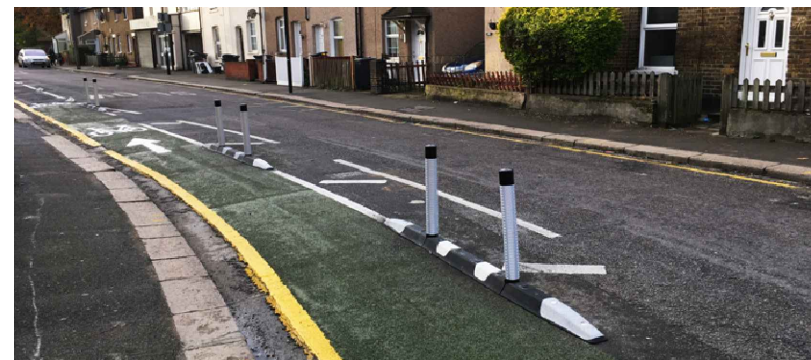
GREENWICH ORCA WANDS - 2.5m LONG SEE DRAWING ARB-12727-1100-01 FOR CONSTRUCTION DETAILS http://www.rediweldtraffic.co.uk/products/cycle-lane-products/greenwich-wand-orca/
