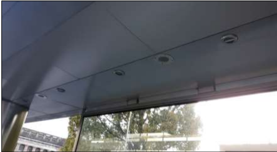
Figure 9: Shelter Lighting (existing design)
