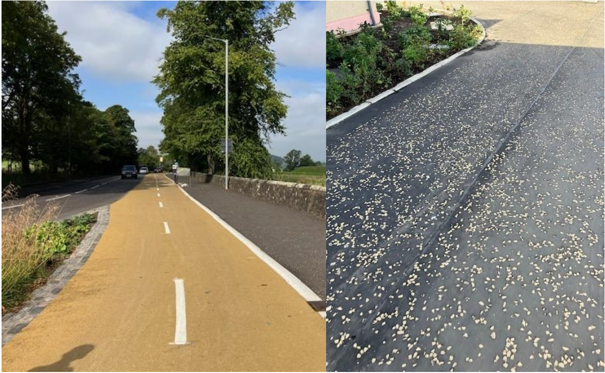
Example of buff surfacing and aggregate in use in Stirling and Longniddry
