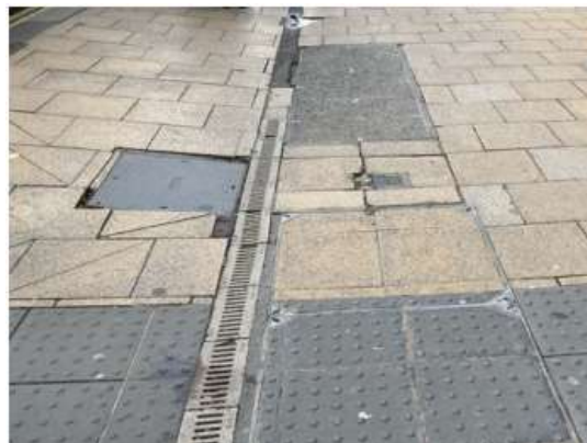
Low quality, easily damaged pavement surfaces
